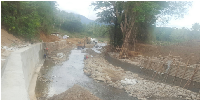
The Department of Public Works and Highways in Biliran is in the midst in constructing two major flood control projects located in Barangay Mapuyo in Kawayan and Brgy. Busali in Biliran town(as shown in photo above)
