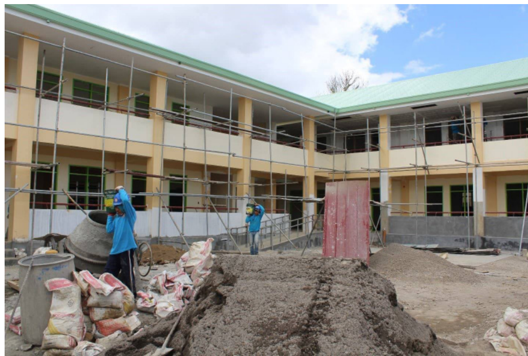
Construction of the 18 classrooms worth P34.4 million, soon to open in Granja-Kalinawan National High School, Jaro, Leyte.
